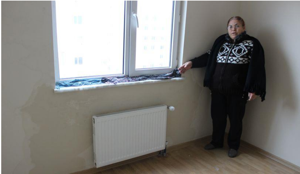
Figure 10-10: The low level of material quality in Kusunlar: when it rains, the water entre the flats. Source: Saltik (2016)
