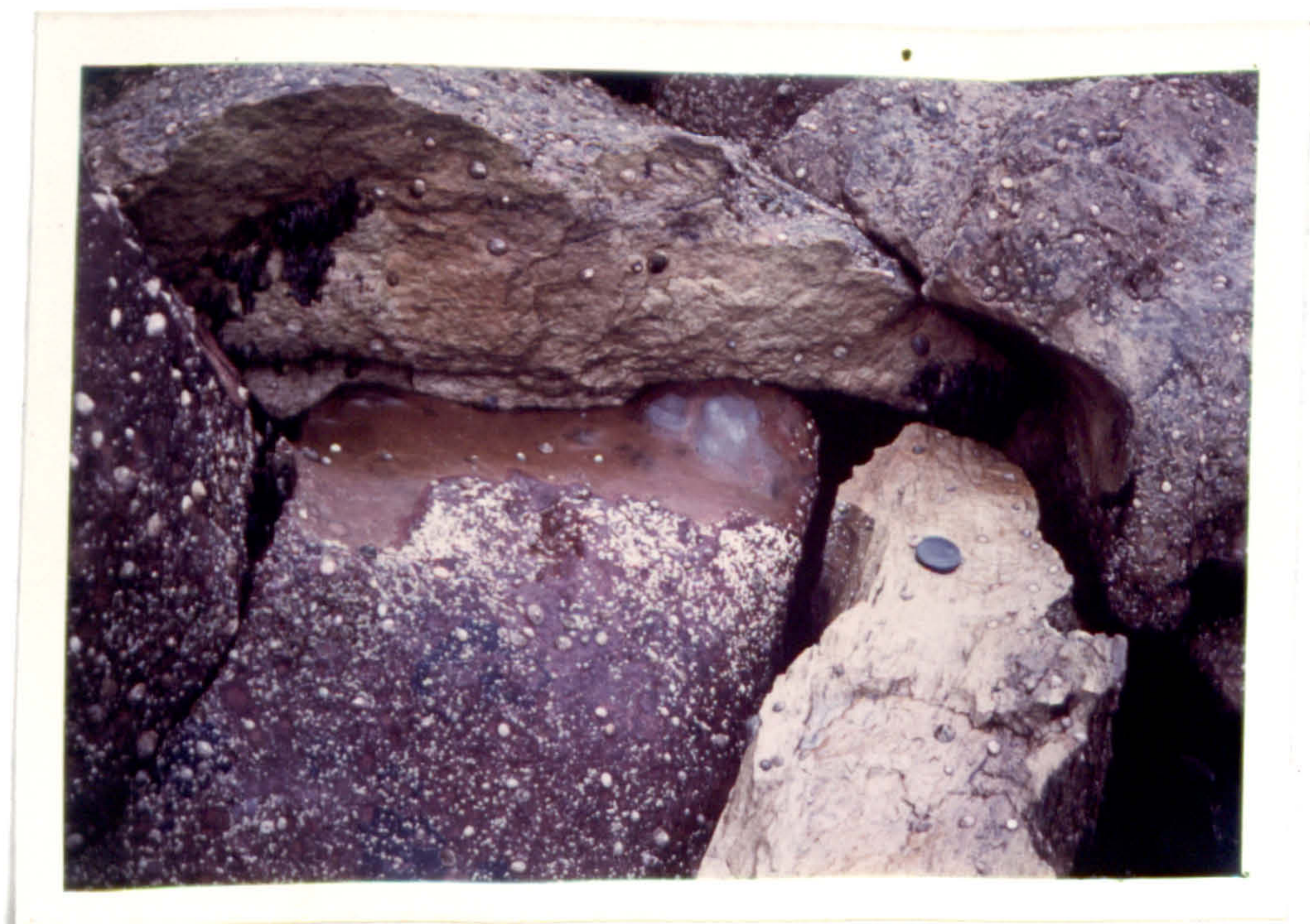
Fig. 6.1b A boulder fractured during a storm
