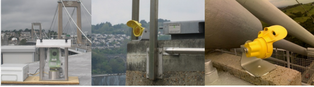
Figure 4.4: Leica TCA 1201M (Robotic total station) located on the South West corner of the roof of the bridge offices and reflectors placed on Plymouth and Saltash side Towers respectively [3].
