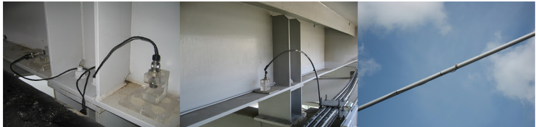
Figure 4.2: Accelerometers placed on deck and cable P4 . From left to right i) horizontal in south deck, ii) vertical in south deck, vertical in north deck and iii) horizontal placed on cable P4 [3].
