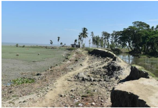
Destruction of soft defence structure by wave actions at Hatiya in the western coastal zone of the country.
