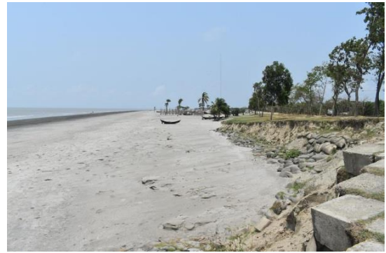
The wave actions at Kuakata coastal area affected the hard defence structure.
