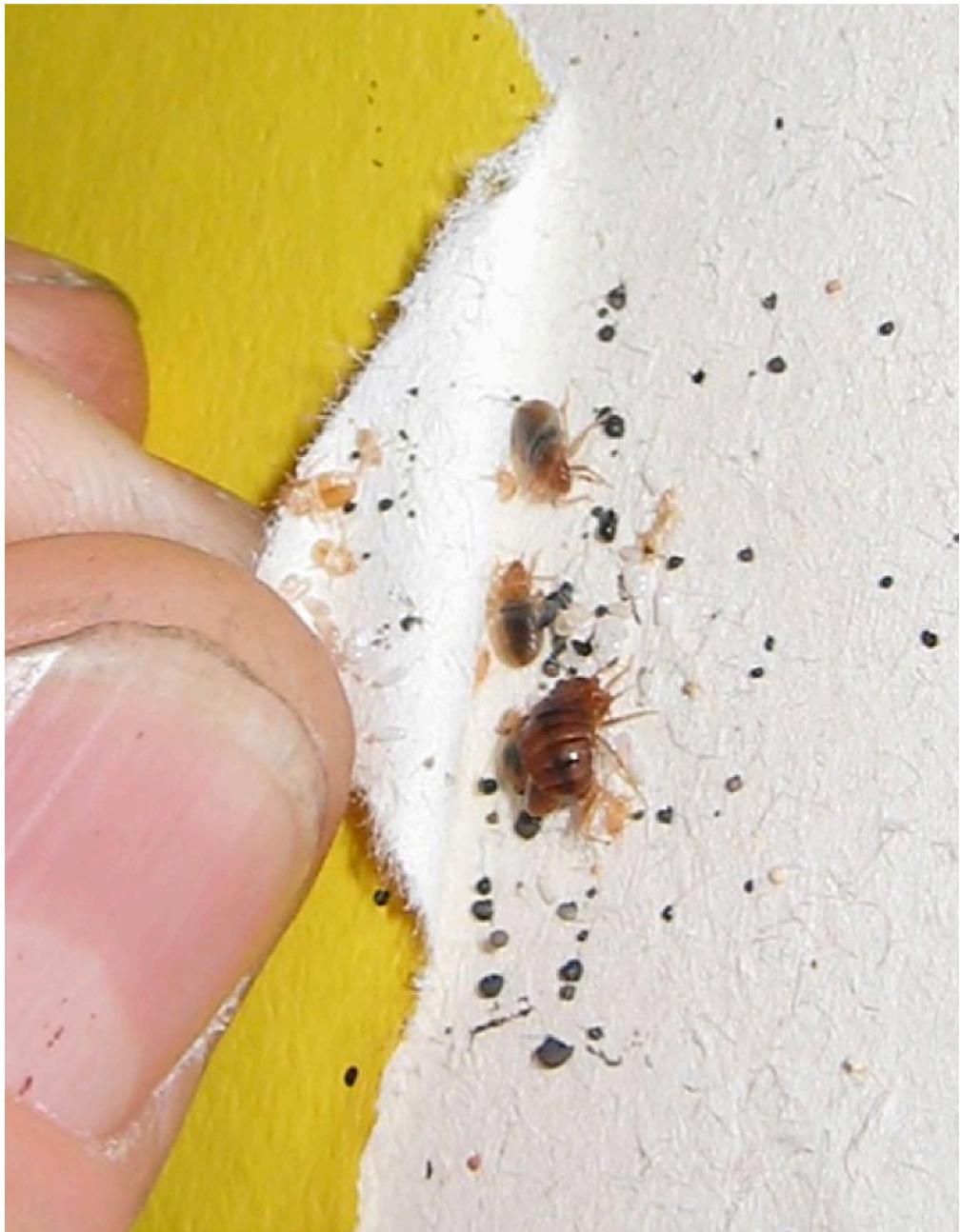
Figure 3.2 shows a typical bedbug harbourage under a flap of peeling wallpaper.
