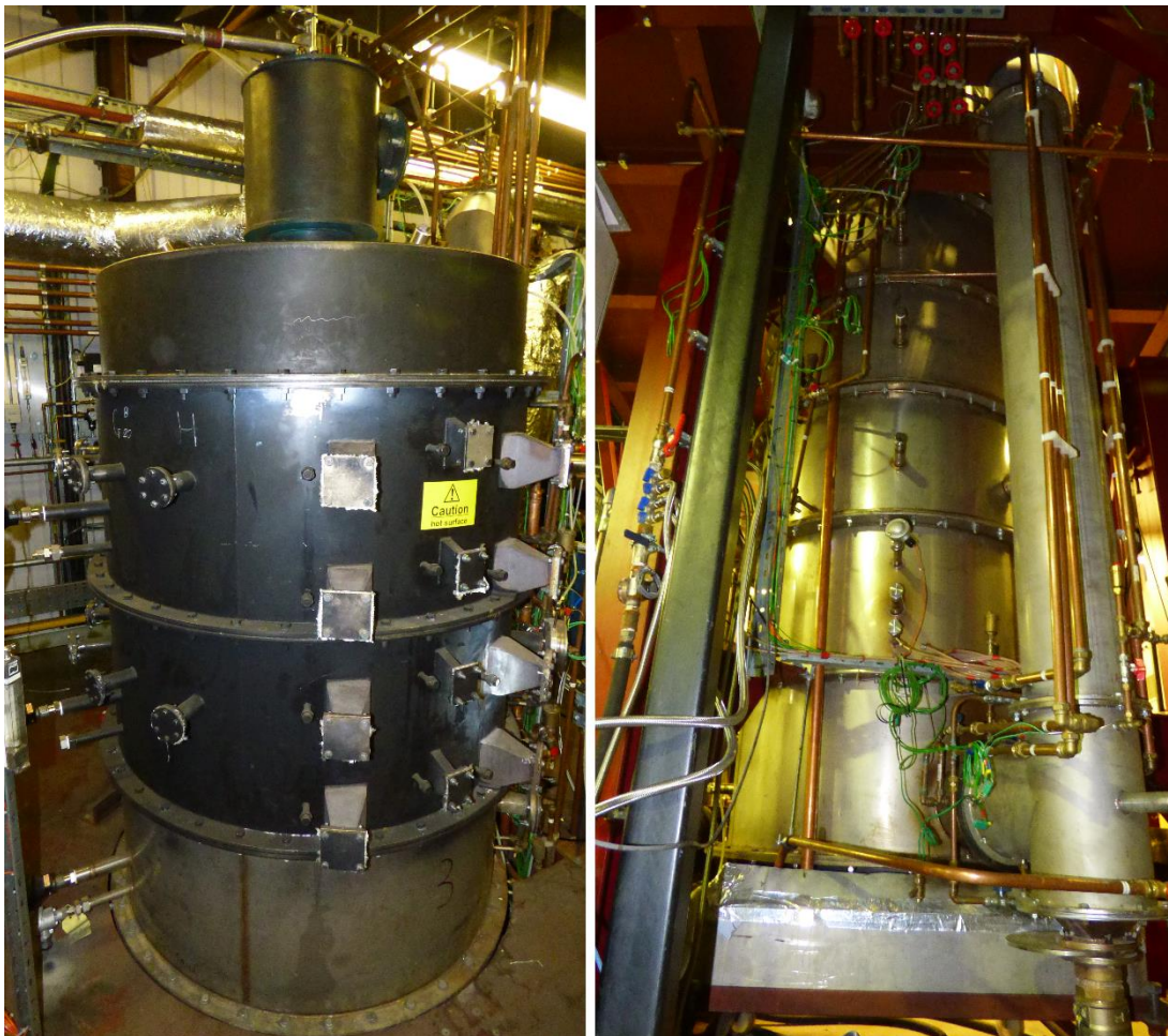
Figure 3.3 Photographs of the 250 kW furnace, the upper 3 sections are located at the mezzanine level (left) while the bottom 5 sections are on the ground floor of the building(right).
