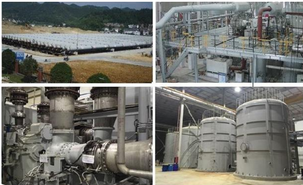
Figure 2-8. A 10 MWe advanced CAES pilot plant (Wang, 2017).
