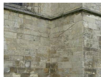
Fig. 55 Roof scars in bay 3 of the cathedral northern aisle
