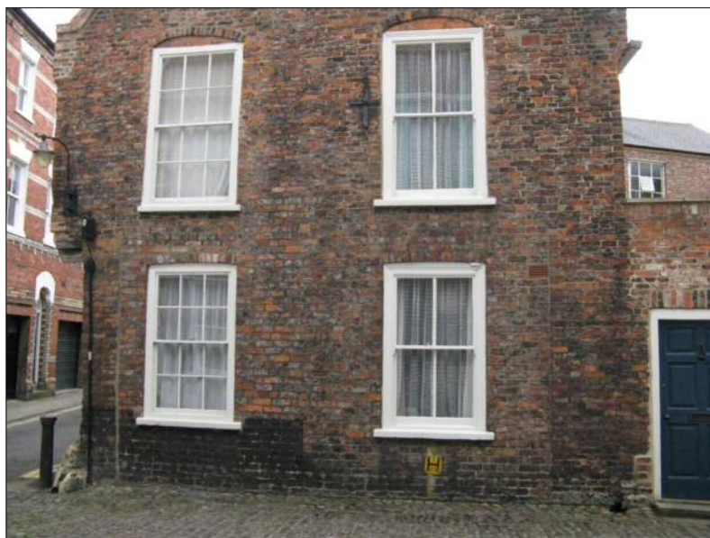
Fig. 41 House in Chapter House Street on the corner with Ogleforth. A vertical wall scar on the left of the front, shows that the building was jettied on both sides.
