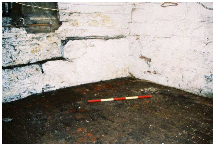
Fig. 114 2 Precentors' Court, north-east corner, showing subsidence towards the right.
