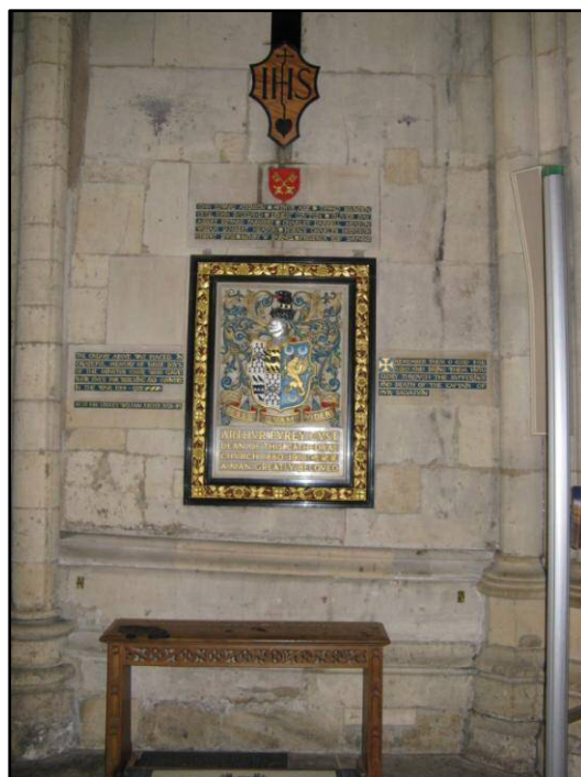
Fig. 103 York Minster south transept, wall between cross aisle and west aisle, first bay . Showing repaired mortise holes.
