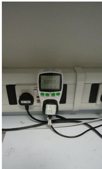
Figure 4-10 The KWh measurement device.
