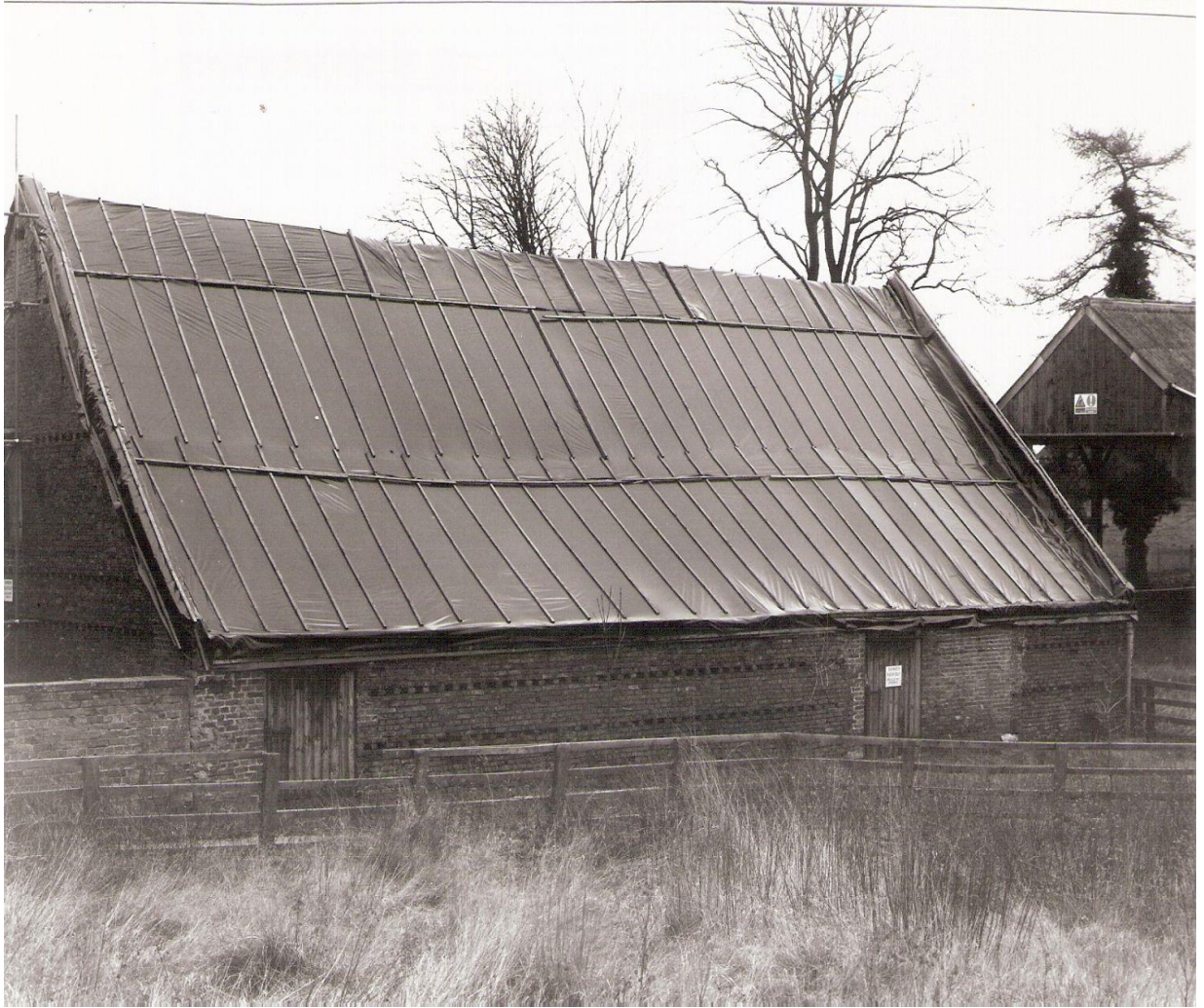
Figure 42. Roof tiles removed by NYCC after some storm damage. Image © Friends of Poppleton Tithe Barn (2016).
