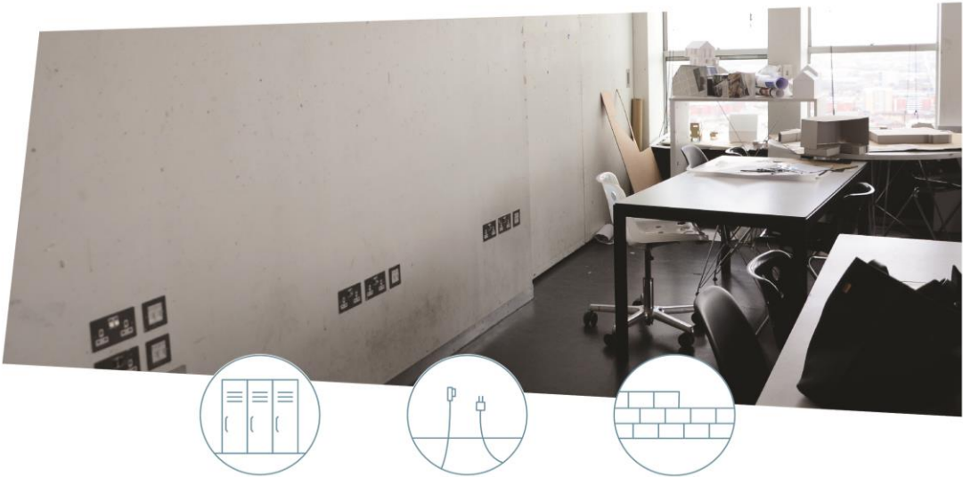
A5 - 72 Power outlets at the only wall in the design studio. Source: Author
