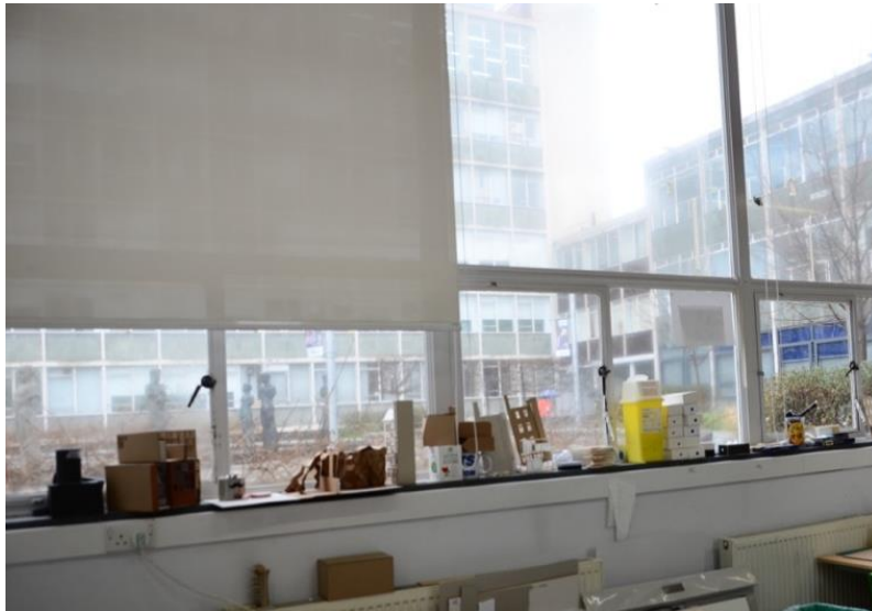
Figure 9 - 9 Items on the ledges of the windows that prevent the blinds from closing at the Northumbria University Design studio. Source: Author
