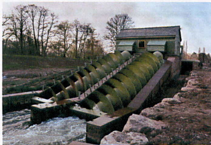
Figure 8.1 An Archimedes screw type microhydro scheme on the River Monnow, Wales. Source: http://www.geograph.org.uk/photo/1538784
