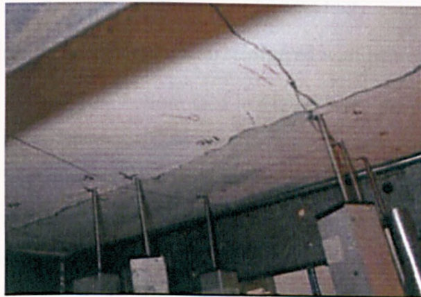
Figure 3.17: Formation of transverse crack.
