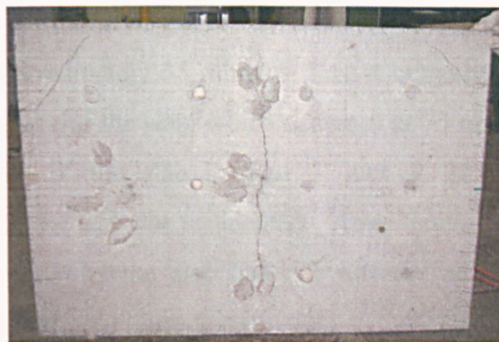
Figure 5.12: View of top face of slab in Test 7.
