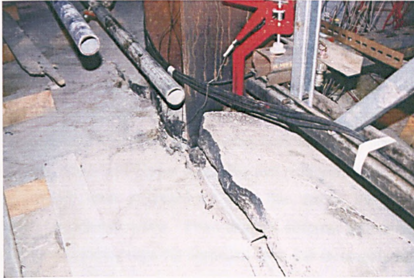
Figure 2.4: Cardington Test 7, photograph of full depth cracking around the compartment edges.
