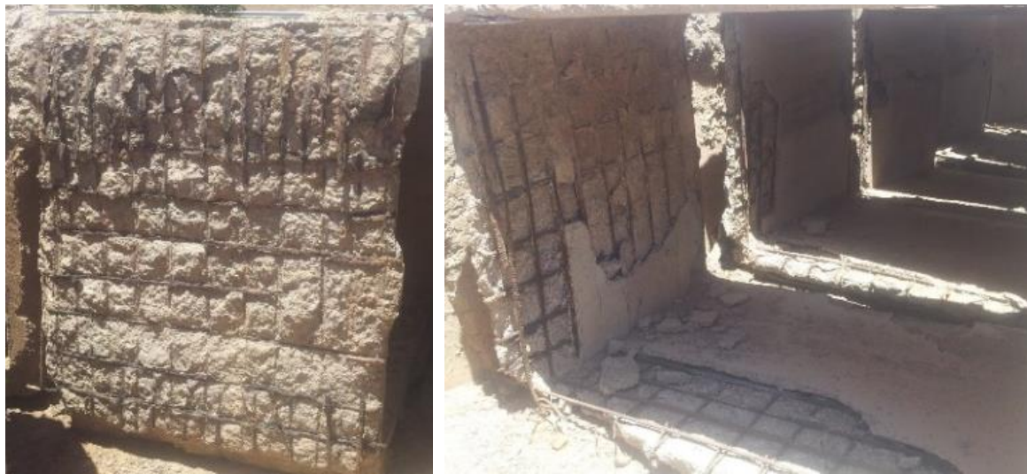
Figure 1.1 Deterioration of culvert boxes (Bahla/Oman-2014).
