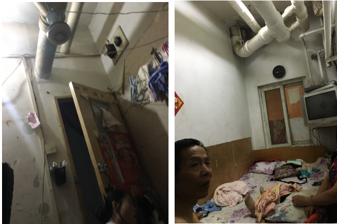
Photo 9-30 Heating pipes in underground basement
