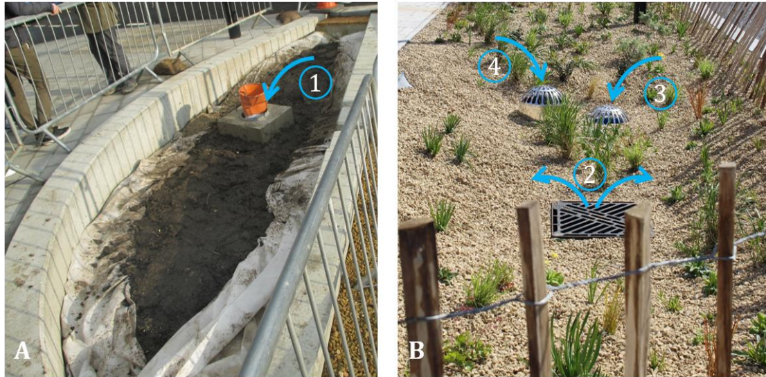
Figure 2.5: Photographs highlighting how outflow is managed on the Grey to Green Scheme.
