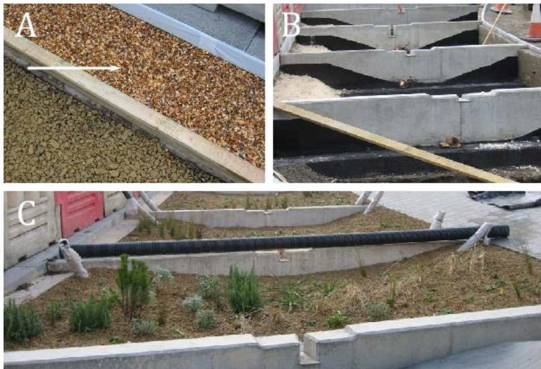
Figure 2.3: Details of the bio-swale elements that make up the SuDS scheme of the Grey to Green (Photographs by author).
