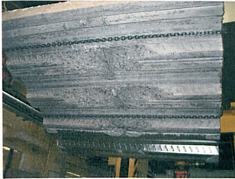
Figure 3.48 Underside of the slab of test PSNM 1-1 showing pull-out failure surfaces
