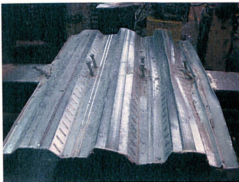
Figure 3.42 The condition of shear studs and steel deck for PTDN 2-1 after concrete slab removal
