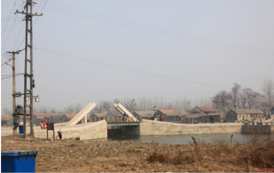
Figure 6.38 The reconstructed Nanyang lock in the Nan Yang section. It can be seen that the lock does not have the correct shape of a canal lock, and components such as the stone crane arms required to control the lock gate are entirely missing; instead, there are four giant concrete objects built with confusion about their function. Information about the substitution cannot be found in any historic records. Such cases raise concerns about the lack of professional knowledge and historical research. Source: photograph taken by author.
