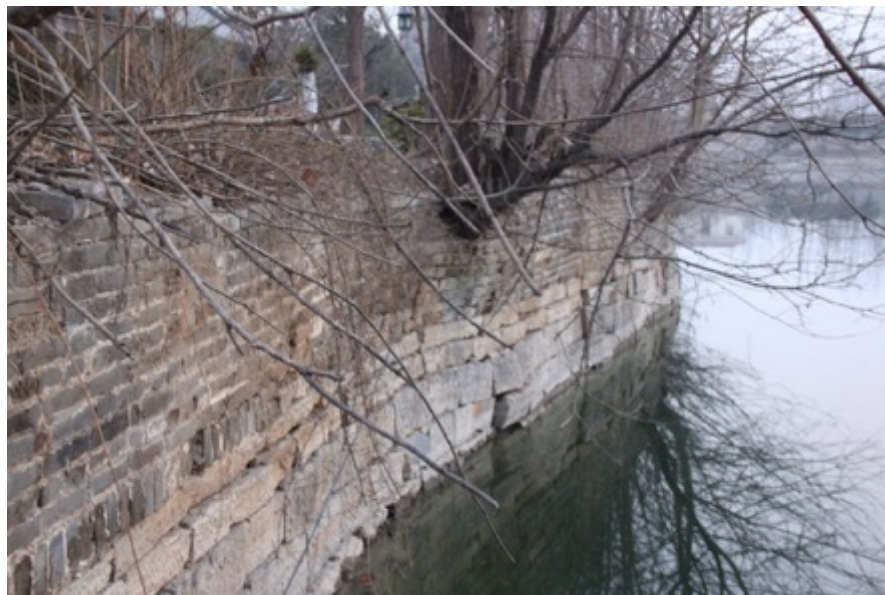
Figure 6.31 This photo by the author shows the original embankment of the Grand Canal in the replica town. Although this is one of the few pieces of original heritage, because of the uneven development of different zones and its relatively distant location, only very few tourists come to or even know about this area, compared to the main commercial streets.
