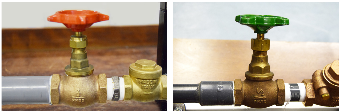
Figure 4.6: Water flow control valves.
