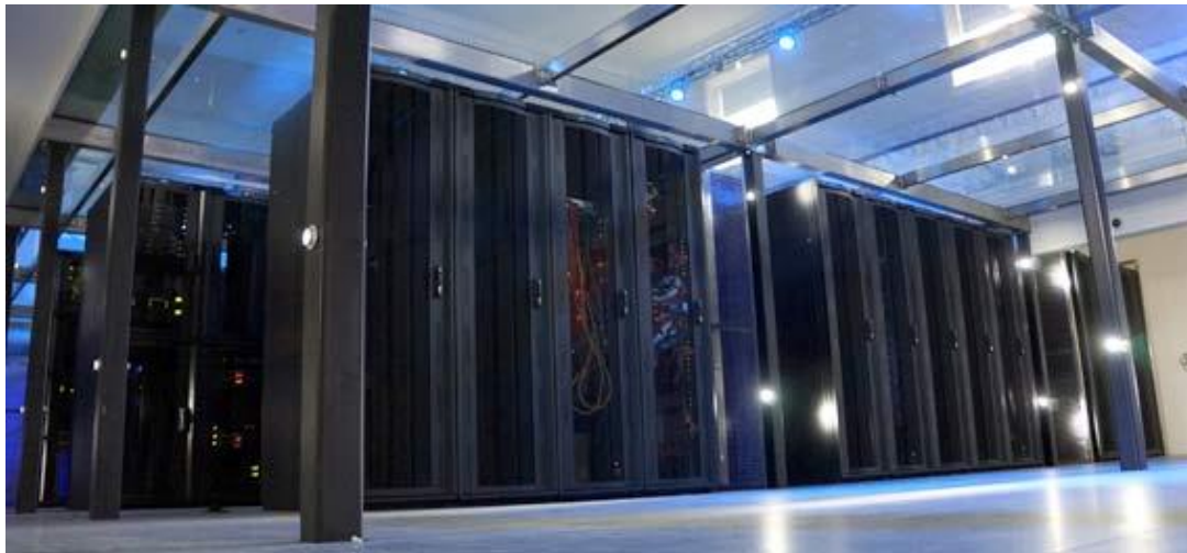
Figure 1-1. Data Centre 3 at aql, a co-location data centre company in Leeds [1]
