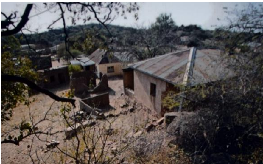
Figure 5.13: Dilapidated kgosi Kgamanyane's house (Source: Bakgatla Heritage Scoping Report)
