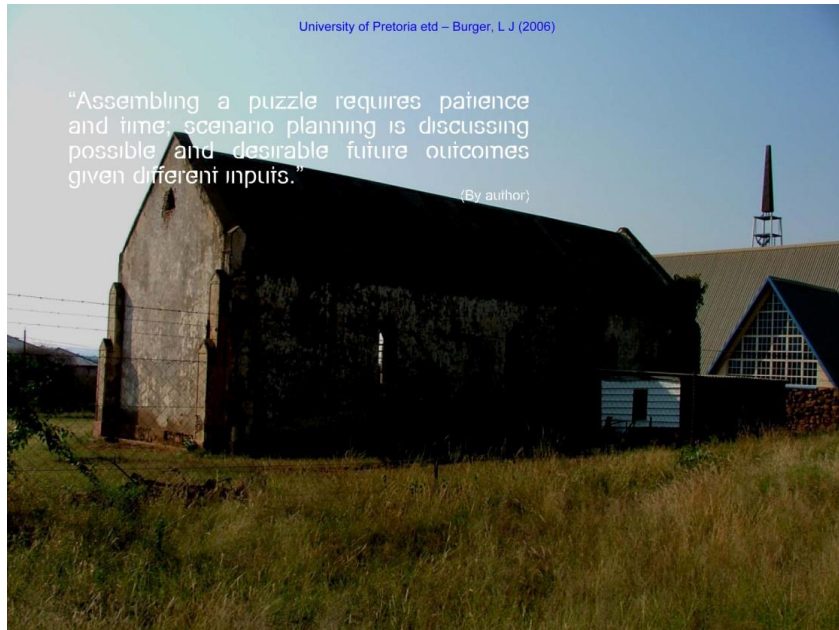
Figure 6.8: Dilapidated DRC church before restoration (Source: Lee Burger, 'Bakgatla-Ba-Kgafela: Design Proposal' (University of Pretoria, November 2006, p 18)
