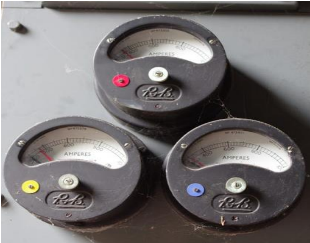
Figure 1-6: A typical secondary substation MDI meters on each phase (SP Energy Networks 2015)
