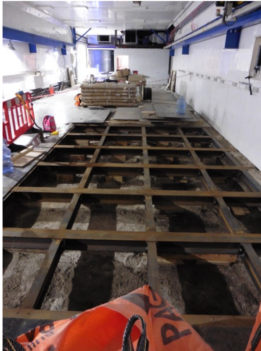
Figure 5.9: Excavation of the rock at Boulby before the installation of the under-floor shielding. (Photo courtesy of S. Paling).
