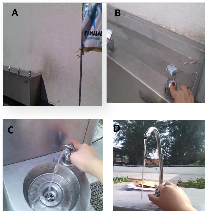
Figure 6-7 Water fountains at intervention sites: not functioning in site A (A,B) and working correctly in site B (C,D).
