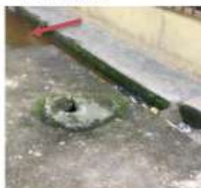
Wastewater leaking from septic tank
