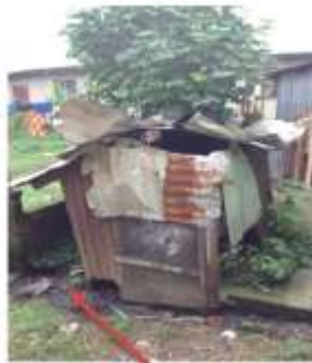
Wastewater discharging from a toilet
