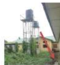
Non-functional water project and ground water above ground
