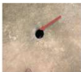
Septic tank with liquid content nearly overflowing
