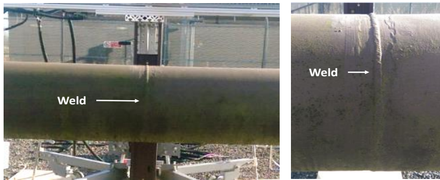
Figure 6.13: NGN 10 in diam pipe showing weld location
