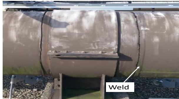
Figure 6.19: NGN 30 in diam pipe showing weld location
