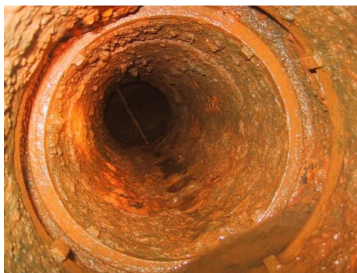
Figure 2-1. Pipeline degradation due corrosion attack [46]
