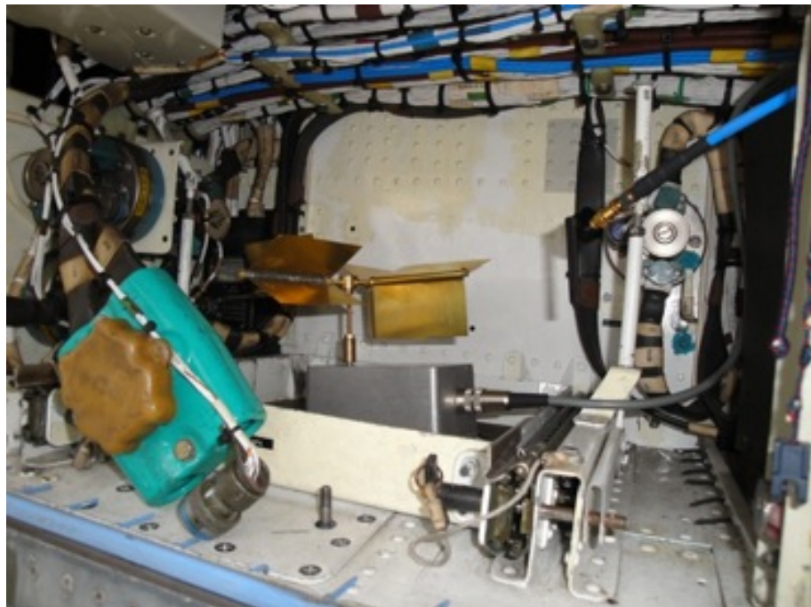
Figure 7.20: The bay used for the more distant antenna in measurement 6
