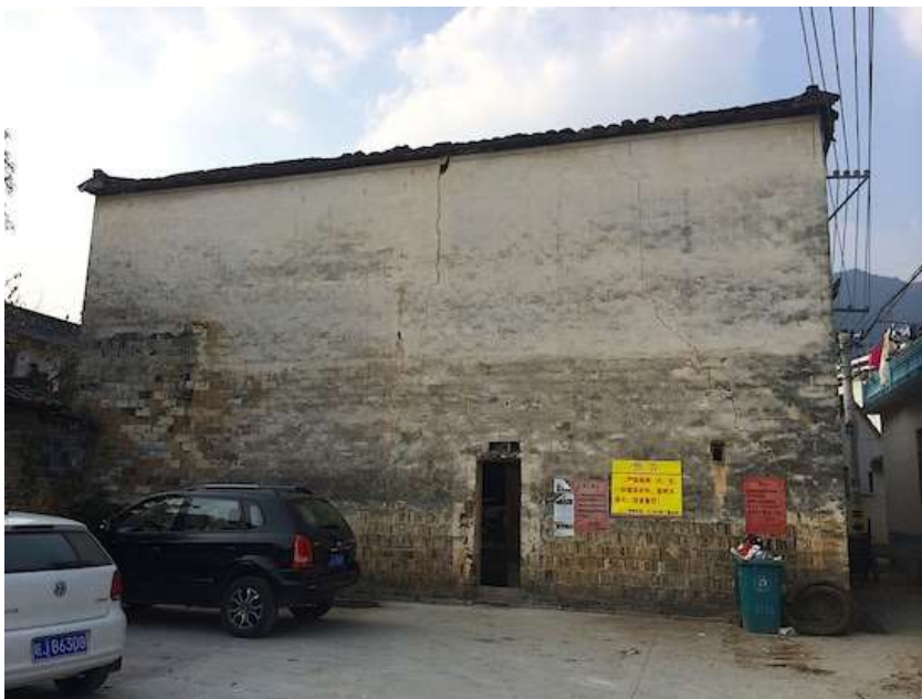
Fig. 7.24 The external condition of existing building to be renovated as 'School of Tillers', Bishan village, November 2014. (Source: http://www.alternativearchive.com/ouning/article.asp?id=945 )
