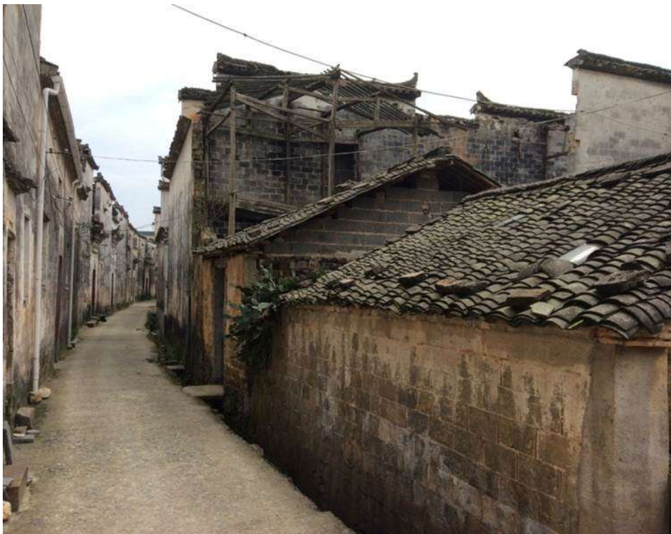
Fig. 0.11 An old building with only a wooden frame was about to demolished in Zhongshan village, which is near Bishan village, Anhui province, China, 2015. (Photographs by the author)
