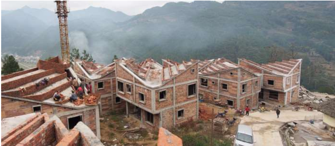
Fig. 3.29 New post-disaster relief houses under construction designed by RUF in Jintai village, Sichuan province. (Photograph by RUF)
