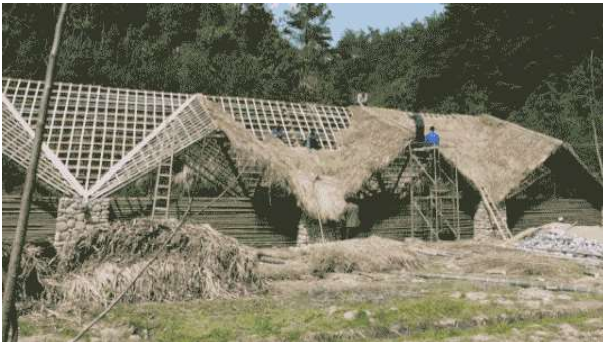
Fig. 5.13 The pig barn was in construction. The rapid and economic construction cost less than two weeks with involvements of much less labour than a normal farmhouse. (Source: Sun Commune)
