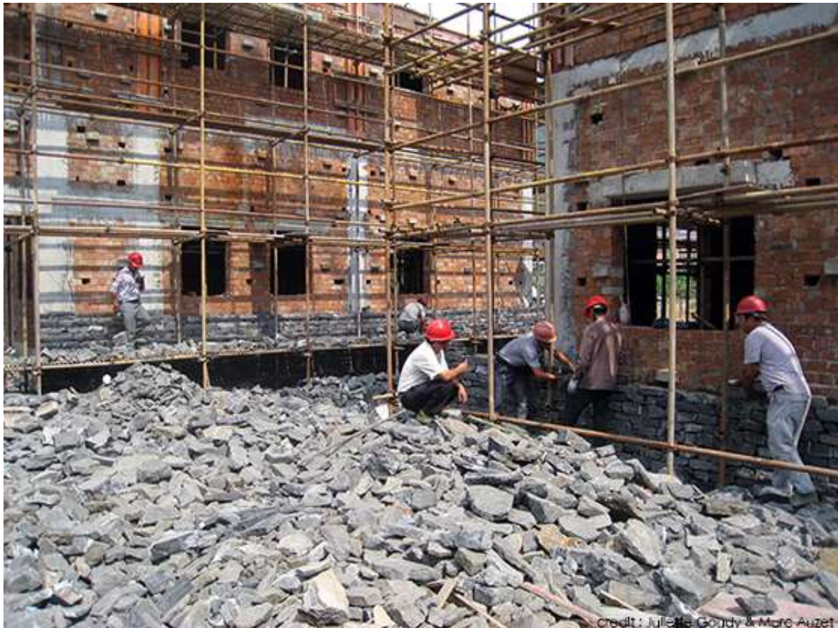
Fig. 6.14 Construction site of new housing (Photograph by Juliette Goudy and Marc Auzet)
