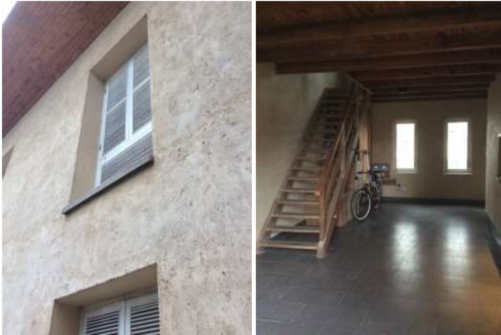
Fig. 8.39-40 Post occupation of Lodge No.3 in 2015. (left) earth skin and window details. (right) entrance foyer and vertical circulation. (Photograph by the author)
