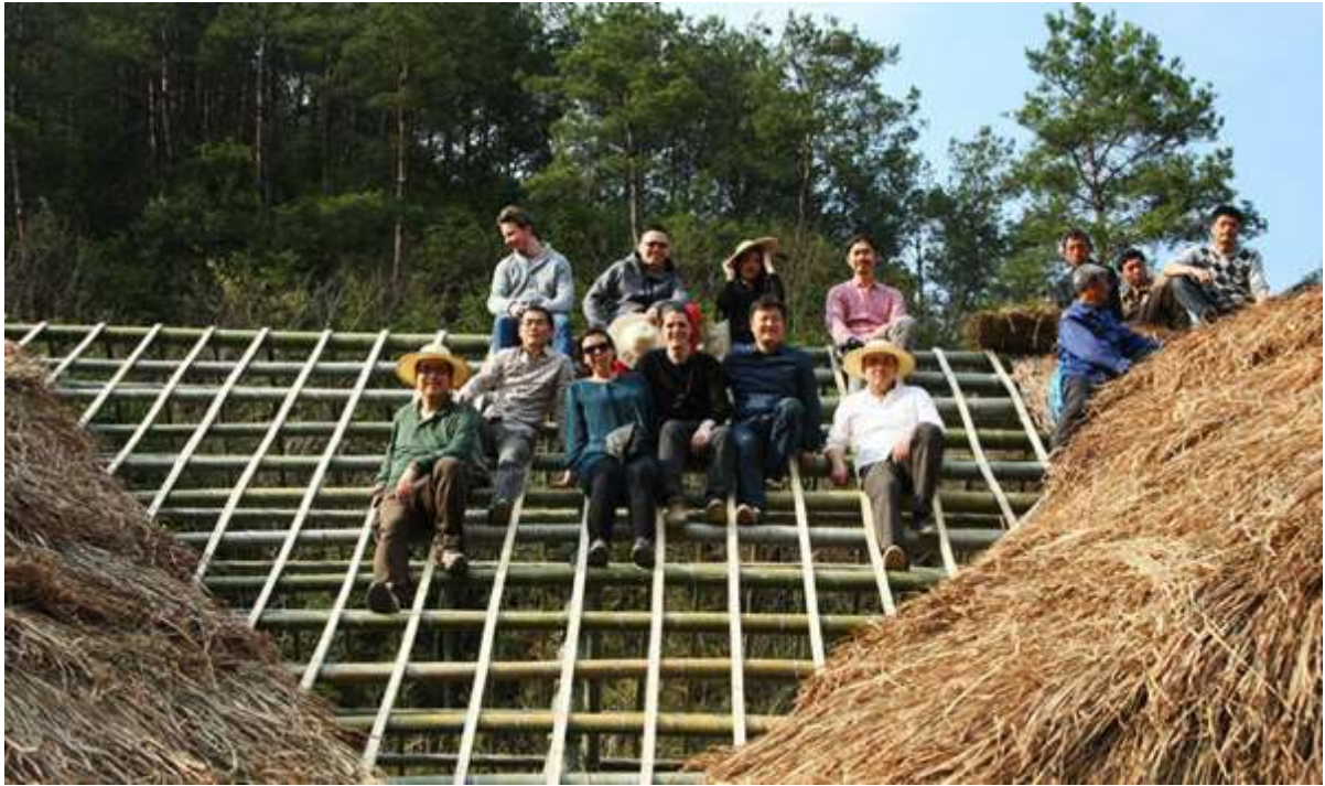
Fig. 5.12 The collective assembly was a joyful process and participants took a group photo on the bamboo frame before the final step for thatch roof. (Source: Sun Commune)
