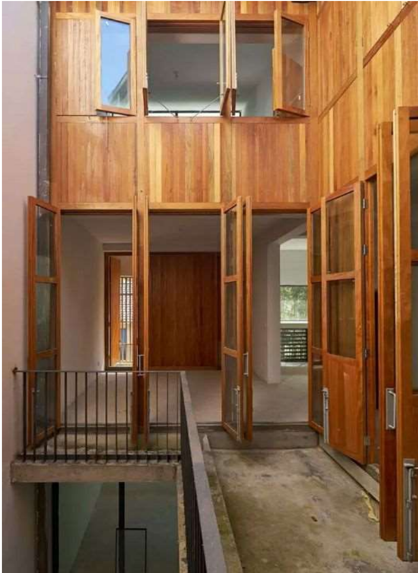
Fig. 6.29 The semi-outside corridor of the first floor of a house has been covered with moss, which made a negative indication that the indoor wooden floor plate might be soon decayed due to lacking of protection from humidity in the design of the courtyard. (Photograph by the author)
