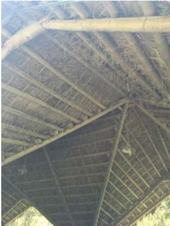
Fig. 5.17 Internal perspective showed the ambiguous practical state between the designed main bamboo frame and secondary structure intermeshed with natural thatch and manmade ductwork providing basic electricity. (Photograph by Wei Song)
