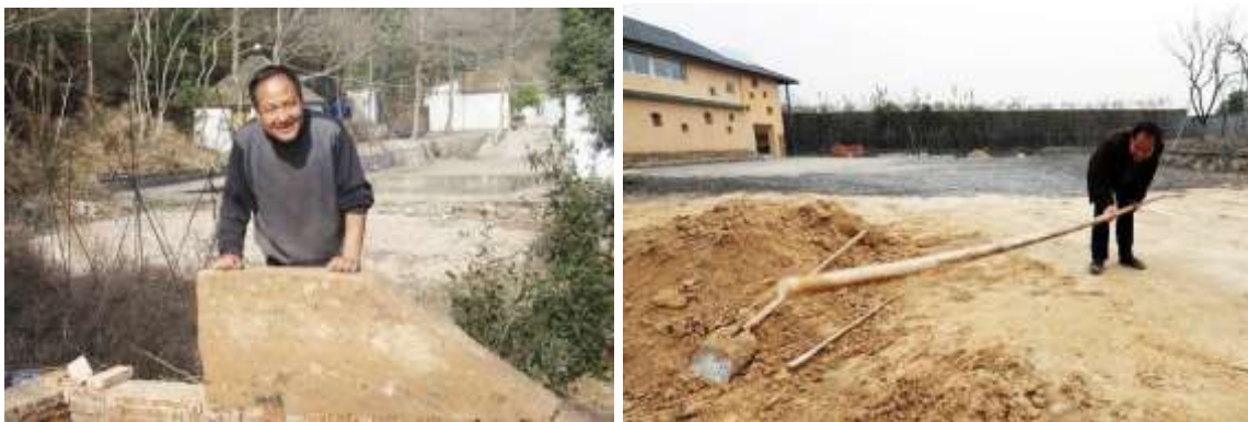
Fig. 8.11-12 Weizhong Ren on design-build site. He used a bamboo pole to beat the earth in order to make it sticky enough for the exterior wall of Eco-lodges. (Photograph provided by Weizhong Ren)
