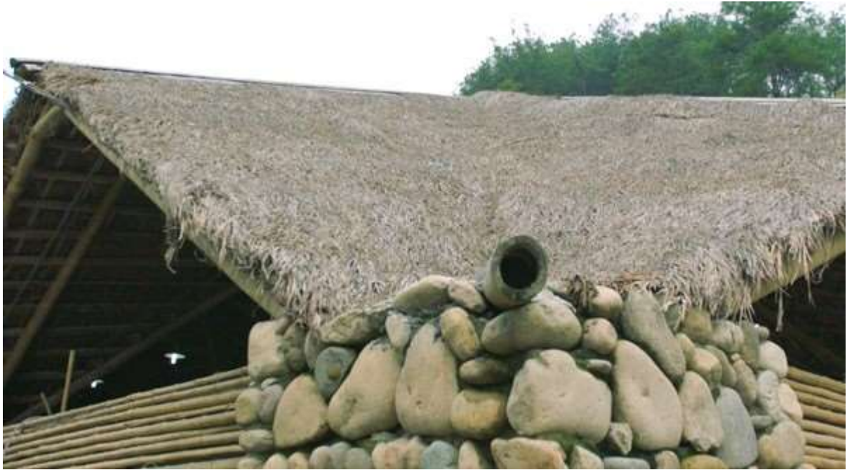
Fig. 5.14 One of the ten meeting points between the bamboo frame and pebbles foundation. No permanent underground foundation was made in order to protect the farmland, therefore the bamboo frame largely depended on its own gravity to keep balanced. (Source: Sun Commune)
