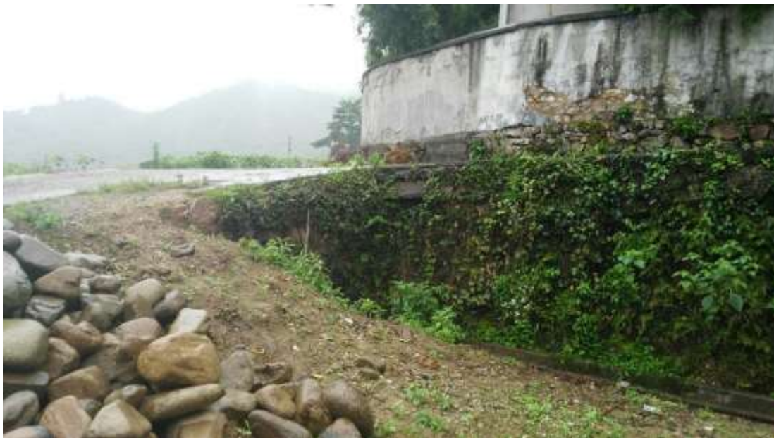
Fig. 9.40 Pebbles as locally-sourced building materials have been prepared on site, 2015 (Photograph by the author)
