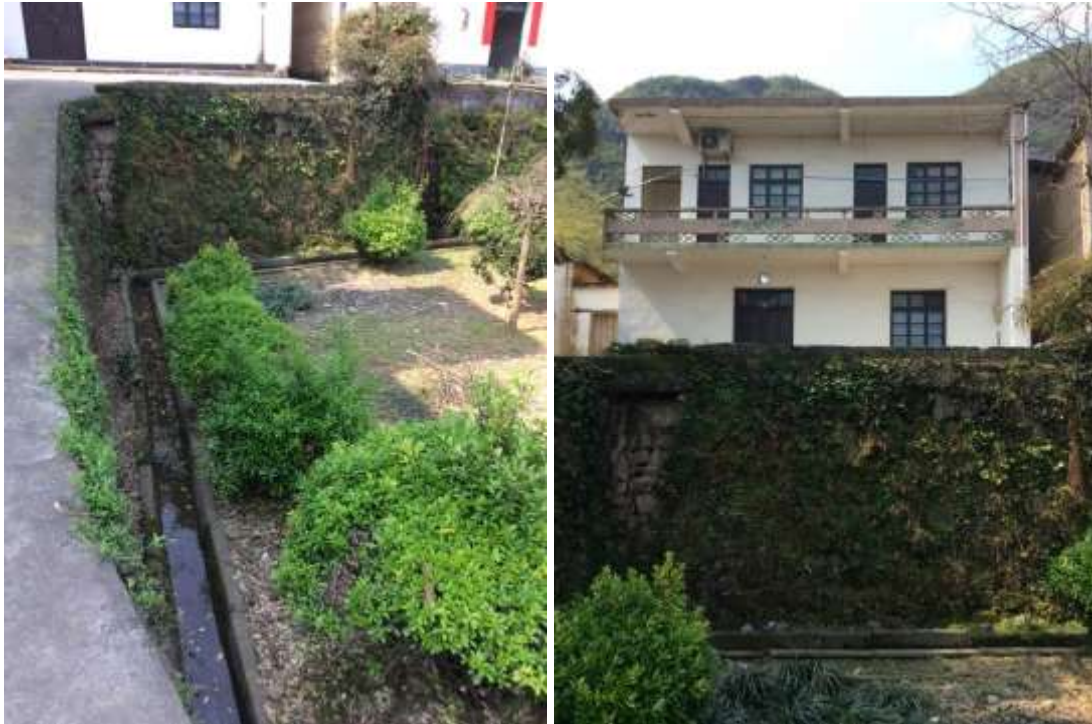
Fig. 9.10-11 Left: Existing water channel for drainage, 2015 (Photograph by the author); Right: Existing retaining wall in masonry, with ecological patches (Photograph by the author)
