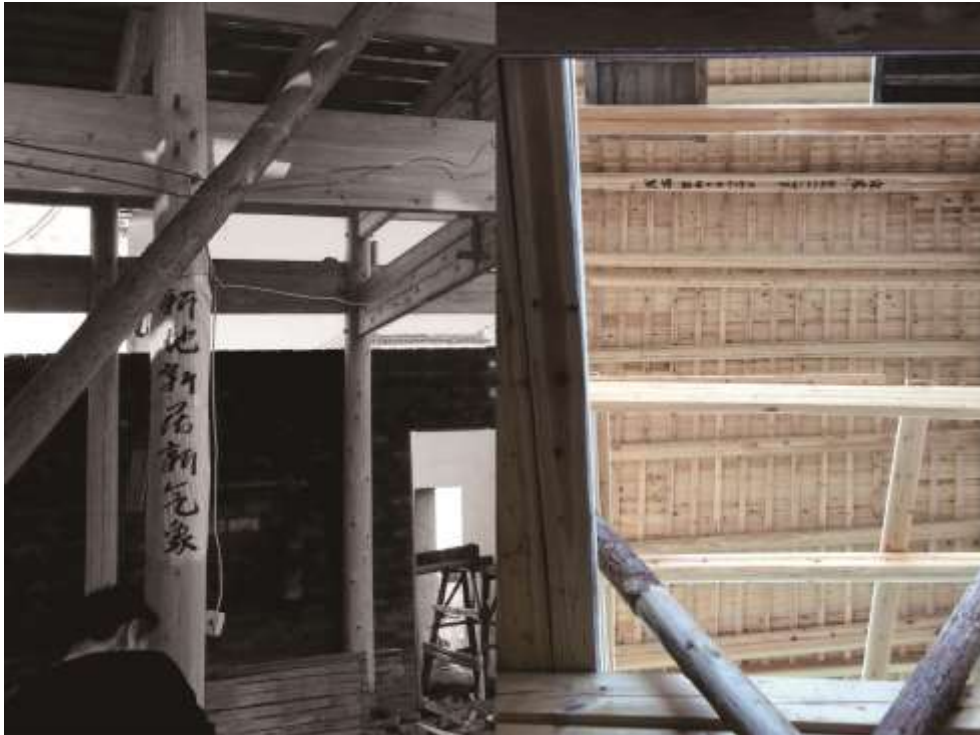
Fig. 3.2-3 Construction of his family house led by one of the last few carpenters in Bishan village, southern Anhui Province, China, 2015. The carpenter-architect had an experience of more than 50 years in building carpentry while without any ability to draw or write architecturally in a modern manner. The textual input from a long-collaborated village gentry was invited in the ritual event of holding up the main beam. All the architecture-related knowledge transfer and collaboration process was through oral instructions in the local dialect. (Photograph by author)
