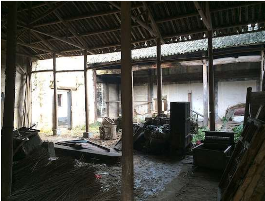
Fig. 7.23 The internal condition of existing building to be renovated as 'School of Tillers', Bishan village, November 2014. (Source: http://www.alternativearchive.com/ouning/article.asp?id=945 )
