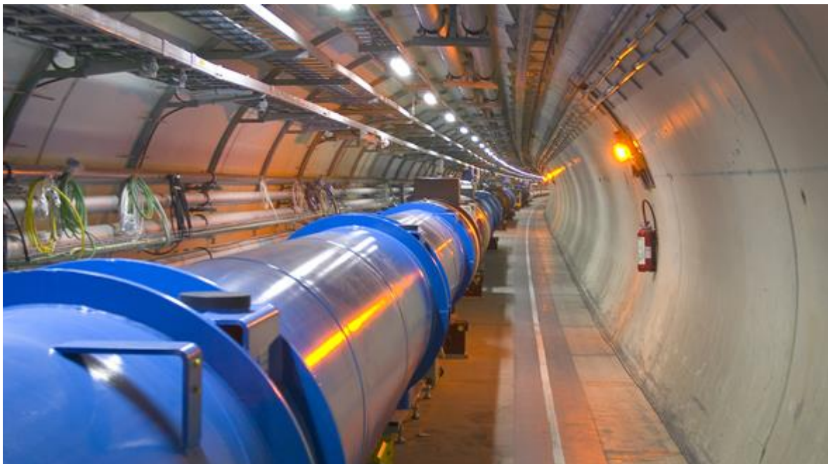
Figure 1-3 Image of LHC Superconducting Magnets [6]
