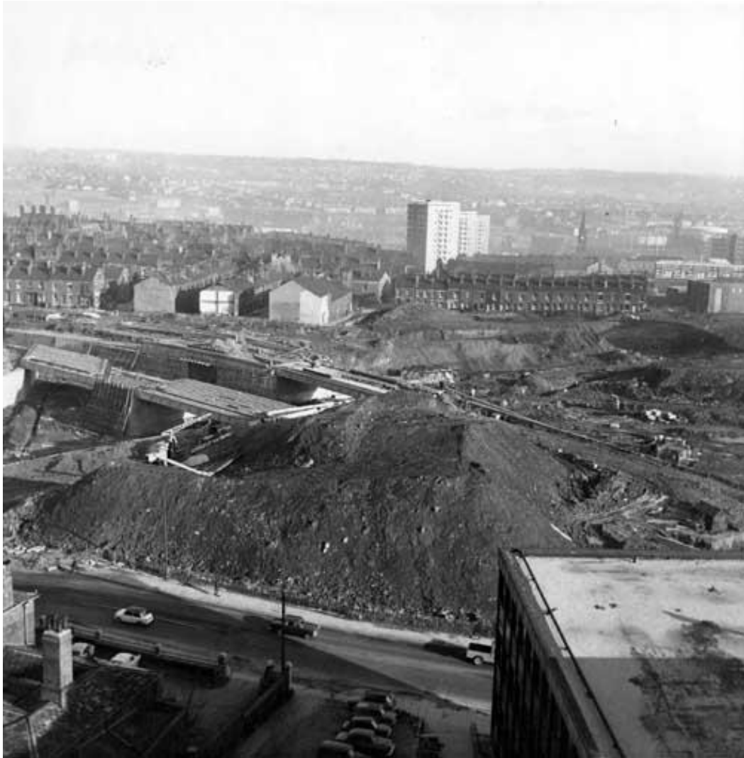
Inner Ring Road construction, Woodhouse Lane, 1965. The houses in the middle distance were also soon to be bulldozed. (WYAS, Leeds, LC/ENG/376/11/no. 1)
