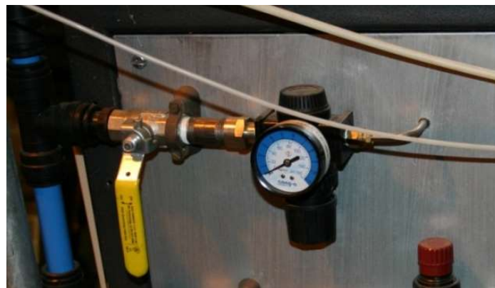
Figure 06: solenoid air supply valve and pressure regulator
