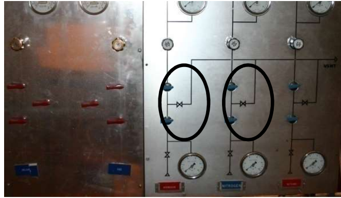
Figure 18: ball valves on N 2 and H 2 line
