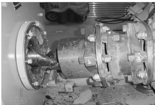
(a) Damaged motor shaft
