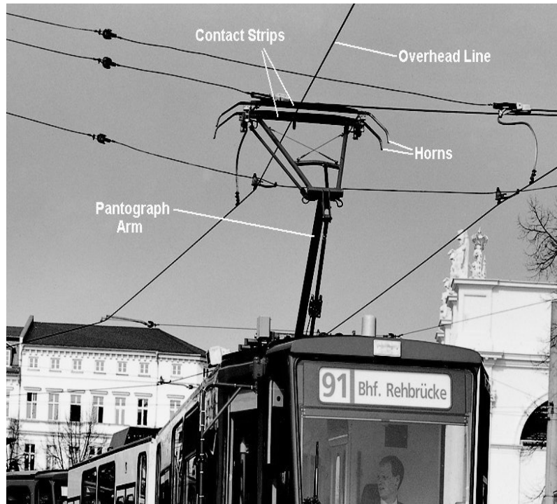
Fig. 2.5 Pantograph-catenary system showing the pantograph arm, overhead line, contact strips and horns 7
