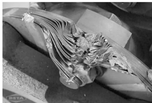
(b) Destroyed coupling
