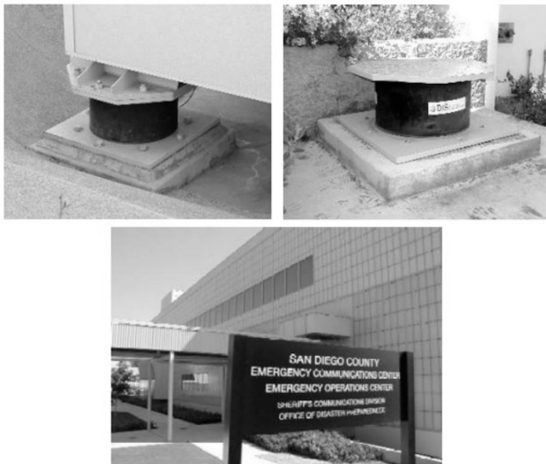
Fig. 1.3 Base isolation in San Diego County Emergency Communications Center 3
