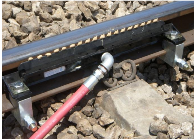
Figure 16: MC4 grease distribution unit in the field.
