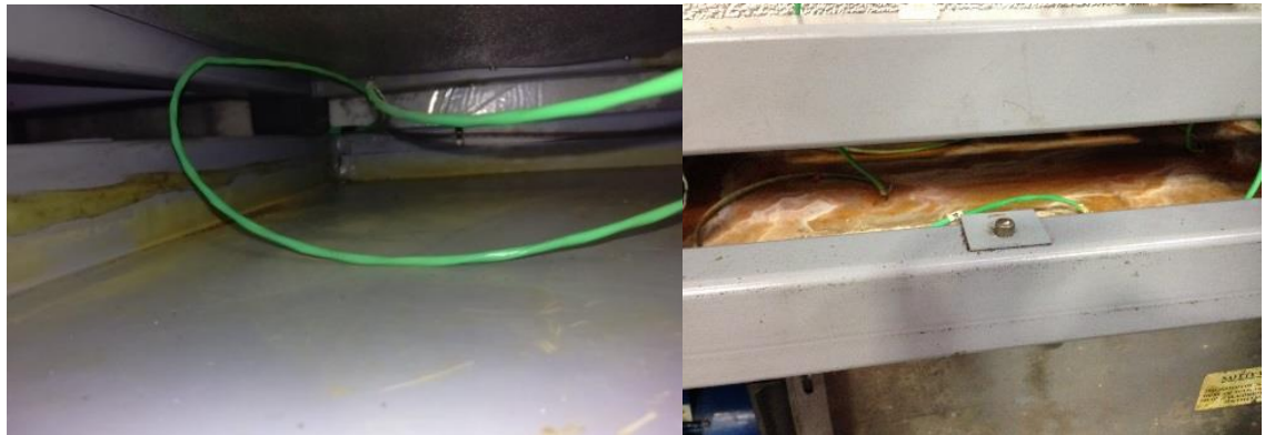
Figure 5-5 Photographs showing evidence of steam condensate rust.
