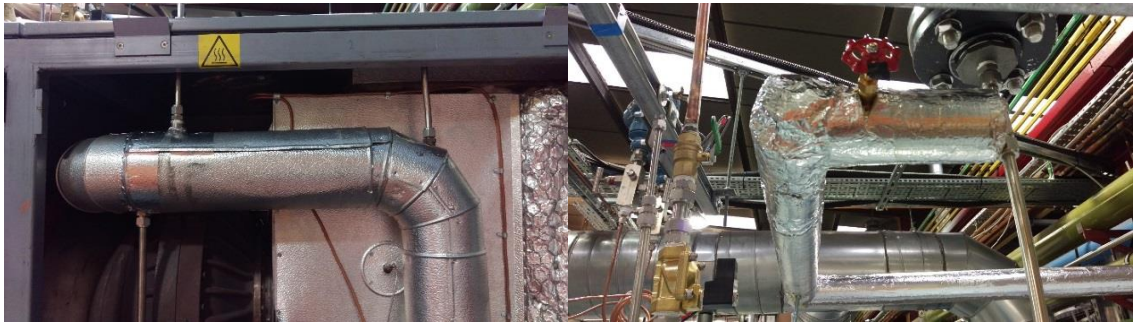
Figure 5-4 Photograph of the steam Injection point into compressed air line, steam deliver valves, manual and pneumatic.
