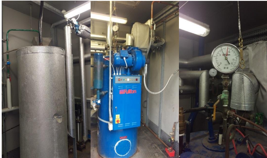
Figure 5-2 Photograph of the boiler house, water tank, boiler, and pressure.
