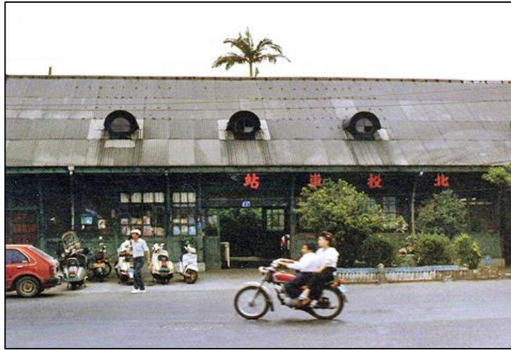
Fig. 5.5 The shabby condition of the Xinbeitou station in the 1970s. The roof has been replaced by corrugated metal roofing sheets. (Source: No author, no date; Accessed Oct. 1, 2016, < http://trstour.com/hsin-pei-tou.htm >)
