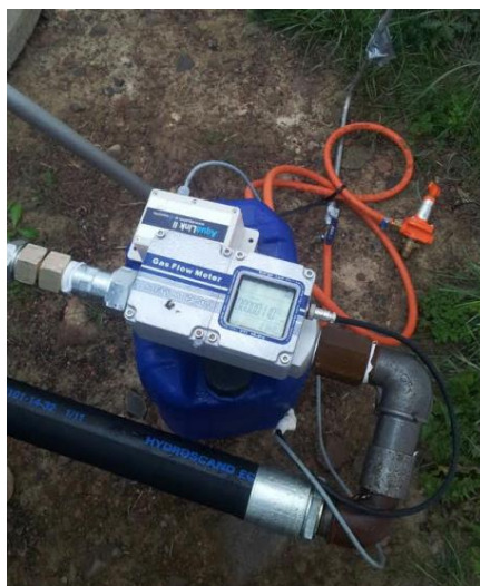
Figure 3.28. Well flow rate measurement system with the SIM card to monitor data remotely.
