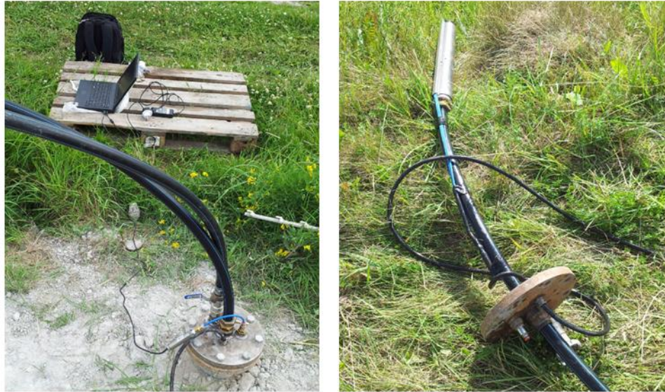
Figure 7.29 water pumping system
