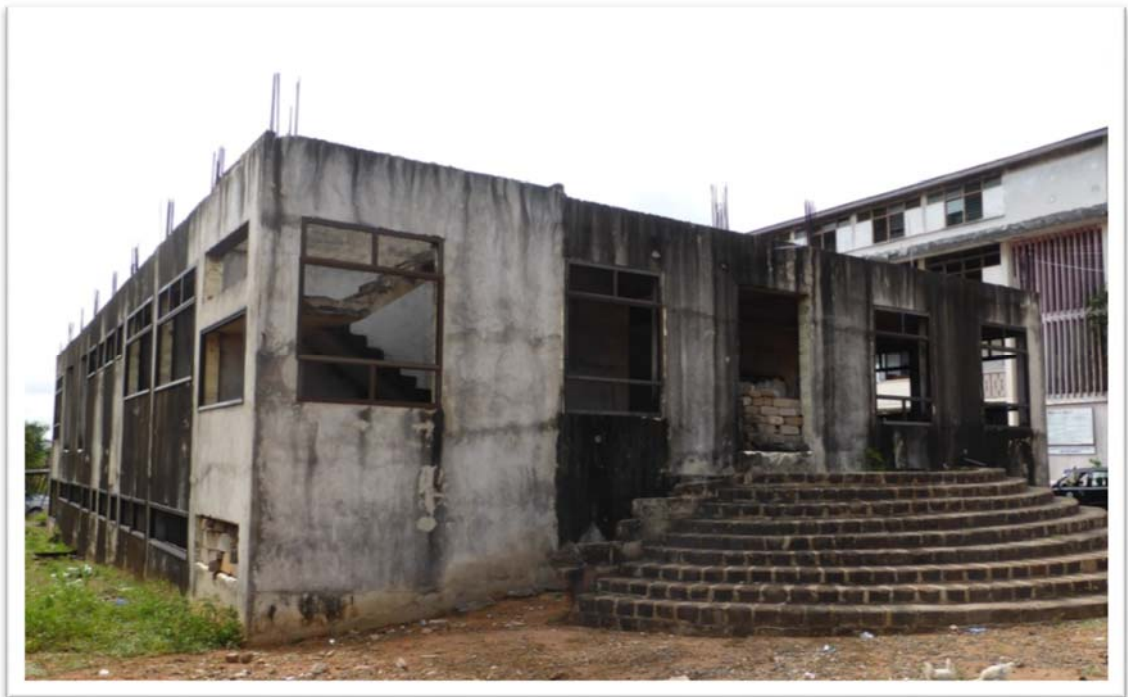
Figure 15 The uncompleted and abandoned building for the Hotel, Tourism and Catering Training Institute
