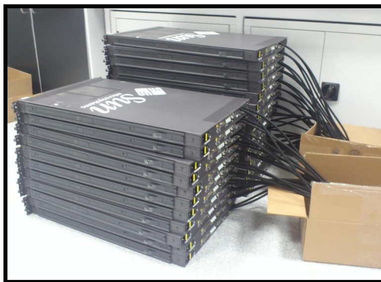
Figure 6.2 Part of the 30 servers with the retrofitted DCLC, Lab1.11, 2013.
