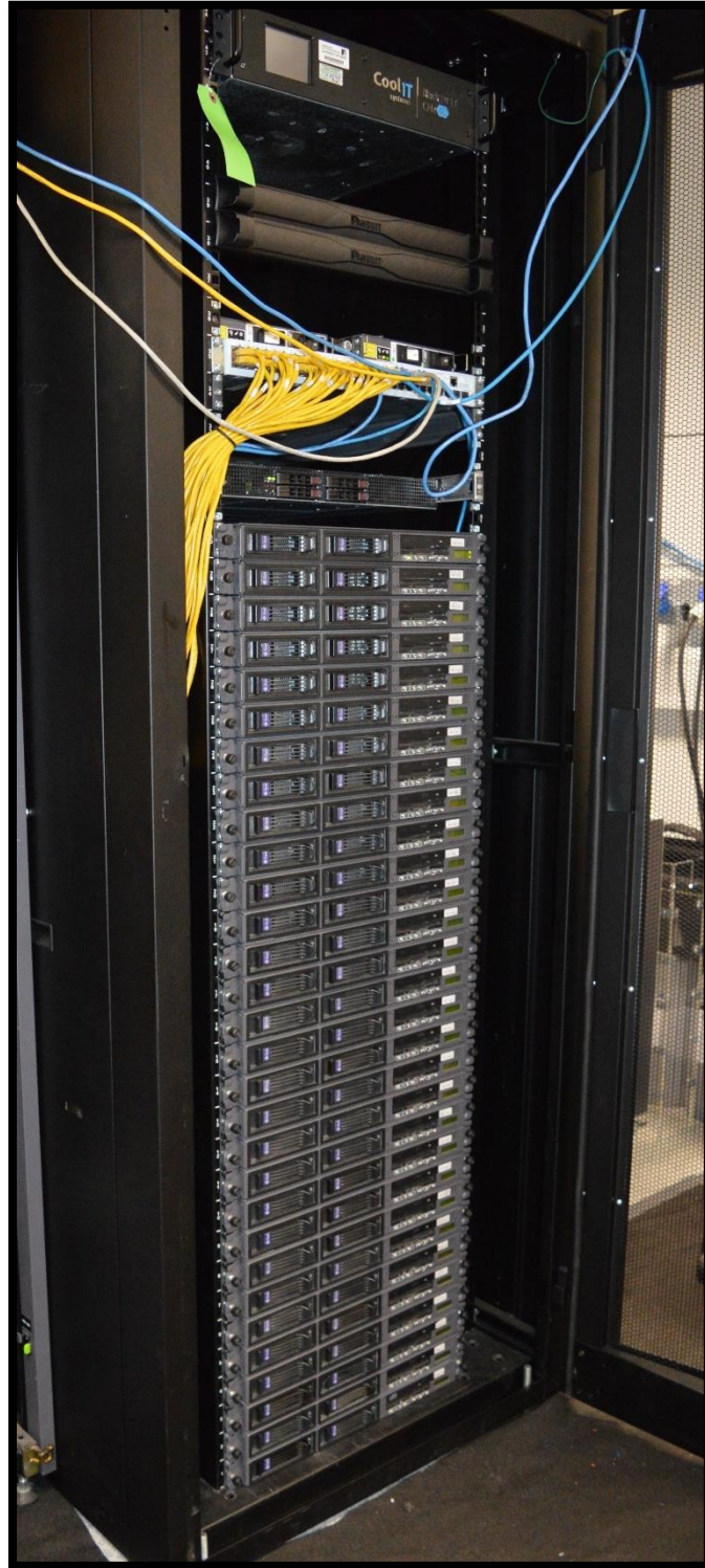
Figure 6.8 The cloud computing rack, Lab 1.11, 2016.
