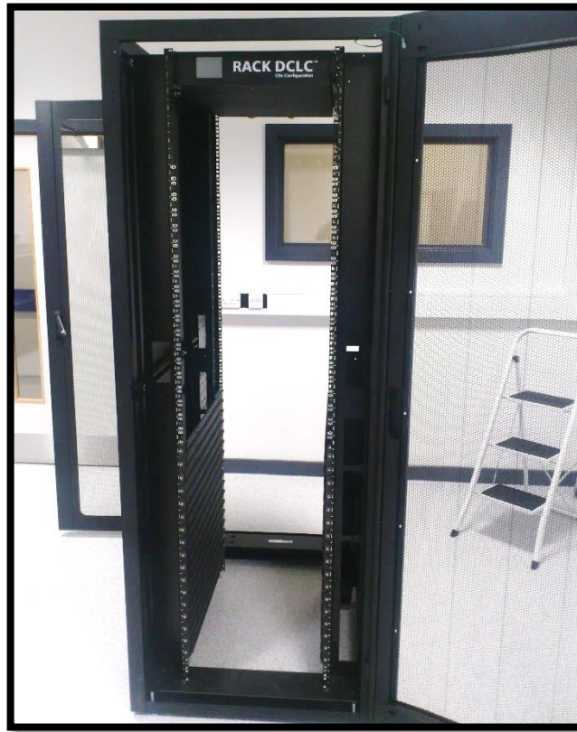
Figure 6.1 The 45U rack during early installation stage, Lab 1.11, 2013.
