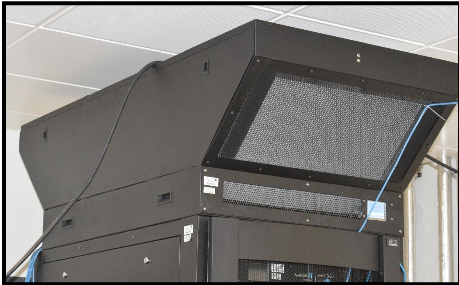
Figure 6.4 The air heat exchanger AHU, Lab 1.11, 2015.
