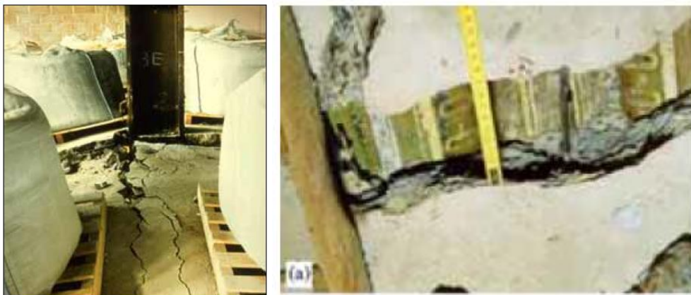
Figure 2.25: Cracked floor slab around the connection [49]
