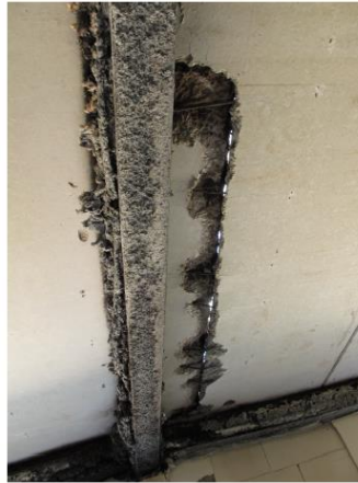
Figure 2.27: Gaping crack, first Munich test [77]
