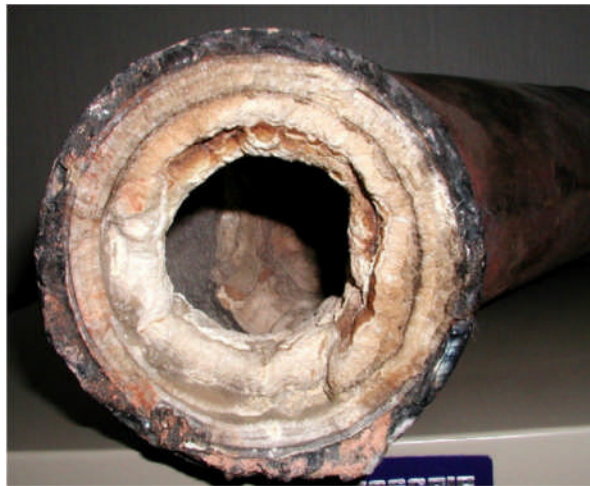
Figure 2.14. Precipitated mineral scale in an industrial pipe (from Baraka-Lokmane and Sorbie, 2010).
