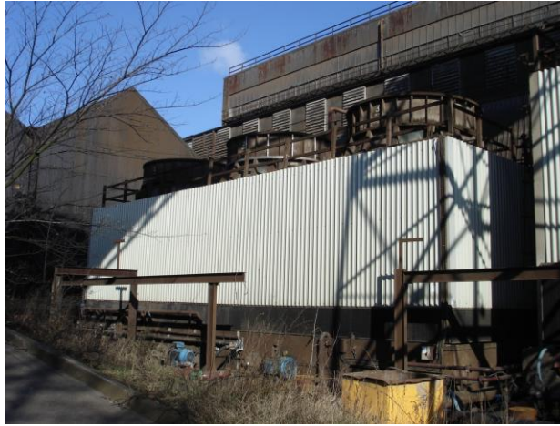
Figure 5-8: The three-cell cooling tower at the back of the Melt Shop. Source: photograph taken during site visit.
