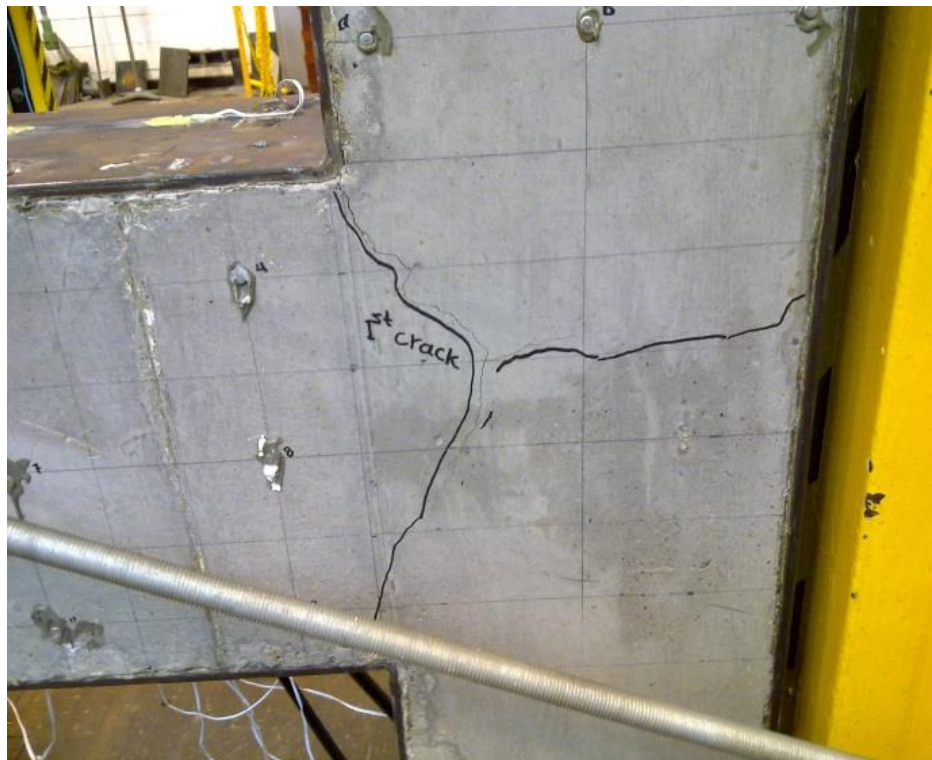
Photo 4-2: First crack in the SCS joint – basic design
