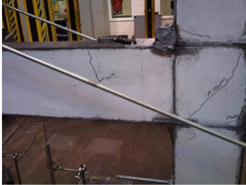
Photo 4-10: First crack in the SCS joint with extended plates
