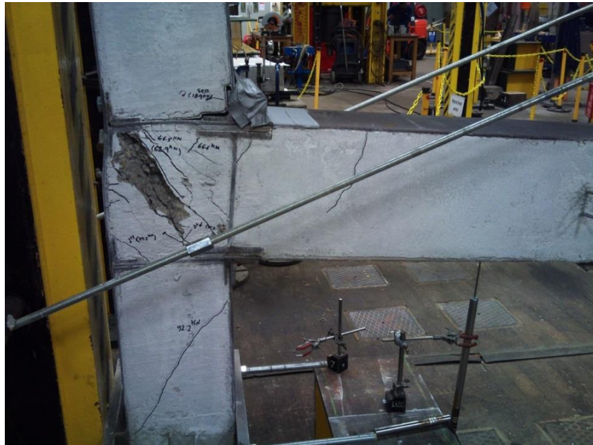
Photo 4-11: Failure of the SCS joint with extended plates
