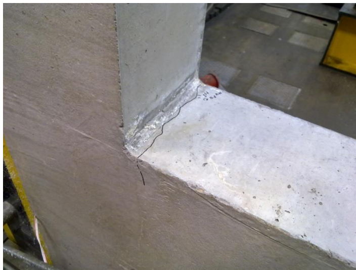
Photo 5-1: First crack location in the RC joint - experimental
