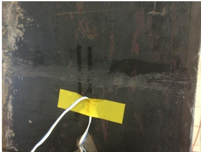
Photo 4-18: Stress concentration at the location of welded studs
