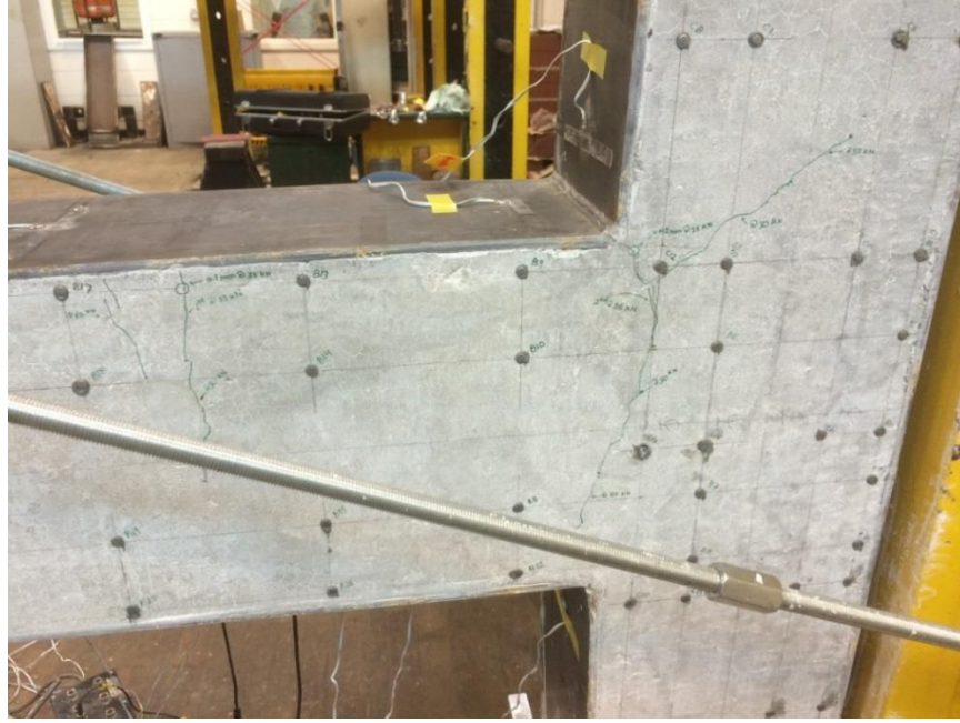
Photo 4-12: Cracking in the SCS joint with HSC
