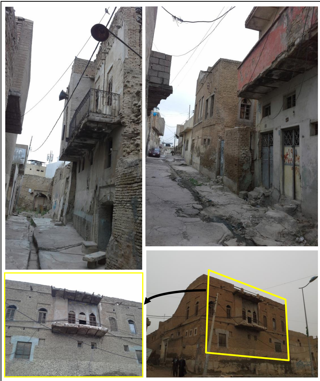
Figure 4.30: Vernacular and heritage single courtyard houses with historical, architectural, and aesthetic values in the area of ‘Sample 1’, and narrow and closed end alleys. The houses have two floors in average. (Source: Researcher)
