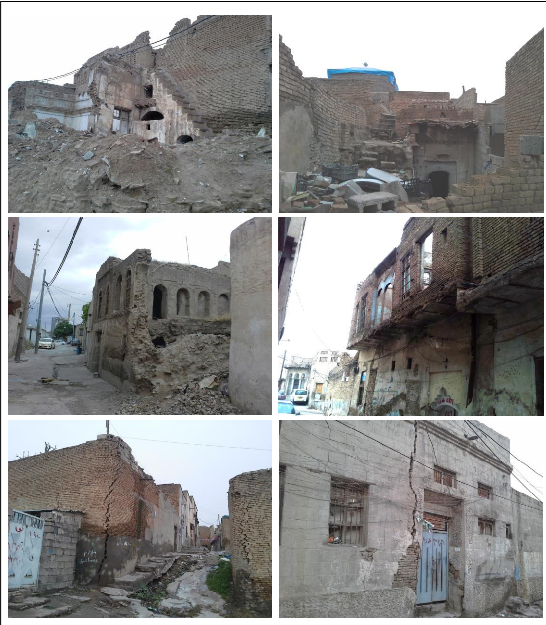
Figure 4.19: Single houses in the area of ‘Sample 1’ (Arab and Taajeel quarters) in a deteriorated condition and they fell down or they are liable to fall down. (Source: Researcher)
