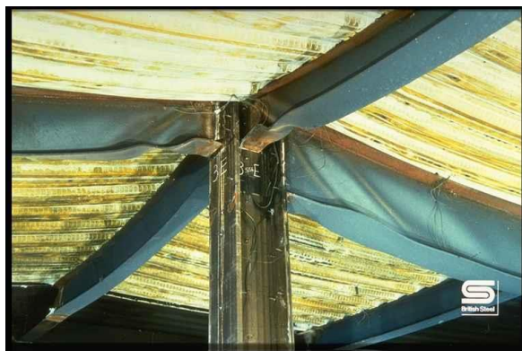
Figure 4-1 Flange buckling and beam-web shear buckling in combination (Newman et al., 2000)
