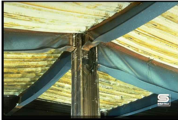
Figure 1-1 Flange buckling and beam-web shear buckling in combination (Newman et al., 2000)
