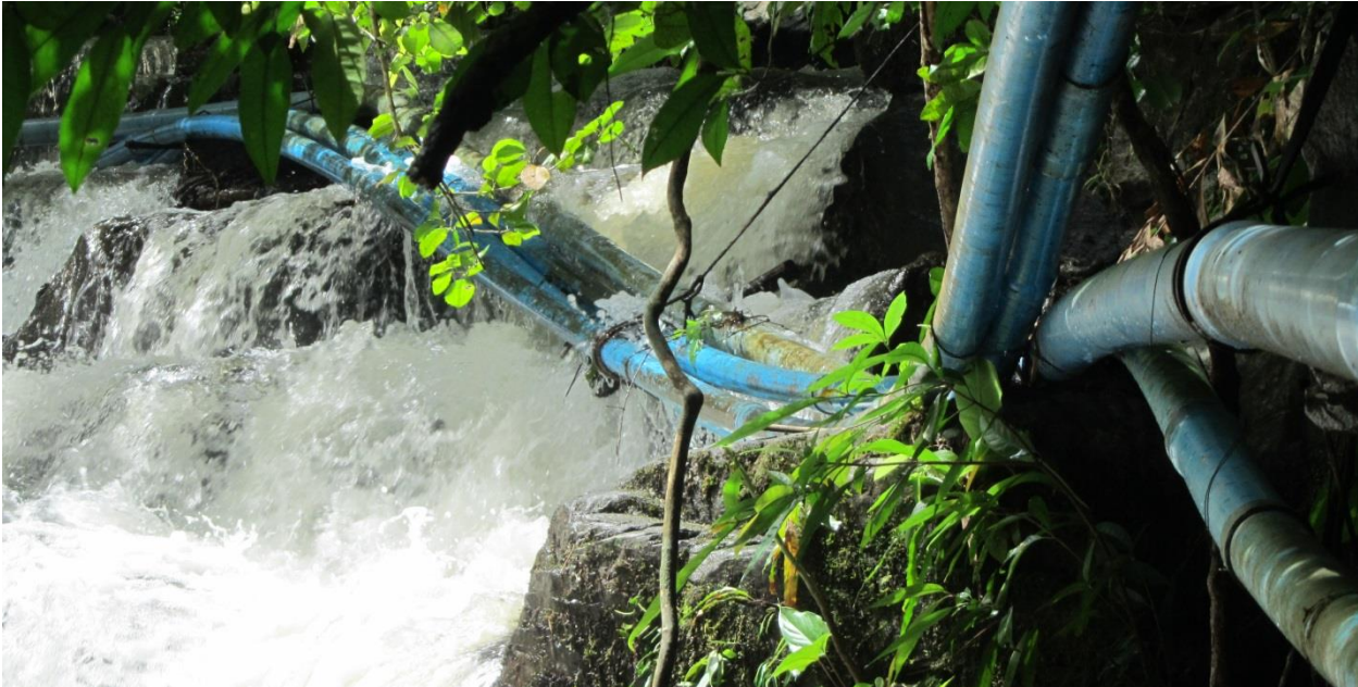
Picture 7.11: Pipes transporting water to the households in Chambok.
