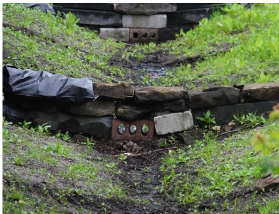
Fig. 5.9. Check dam with drainage holes at bottom. Photo was taken by the author in August 2014.
