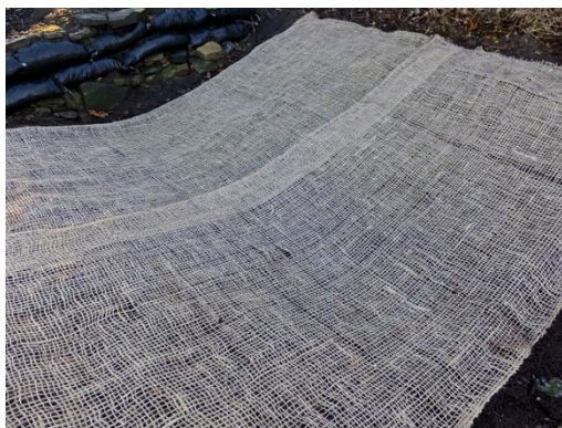
Fig. 5.30. Hessian erosion control mat pinned over the top in every experimental unit to hold soil in place. Photo was taken by the author in December 2013.
