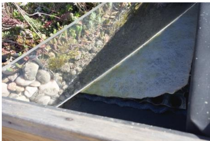
Fig. 2.6. The typical multi-layered green roof system (from top to bottom: vegetation, growing medium, filter mat, water storage and drainage layer, root barrier and waterproof layer). Photo was taken by the author in June 2013.
