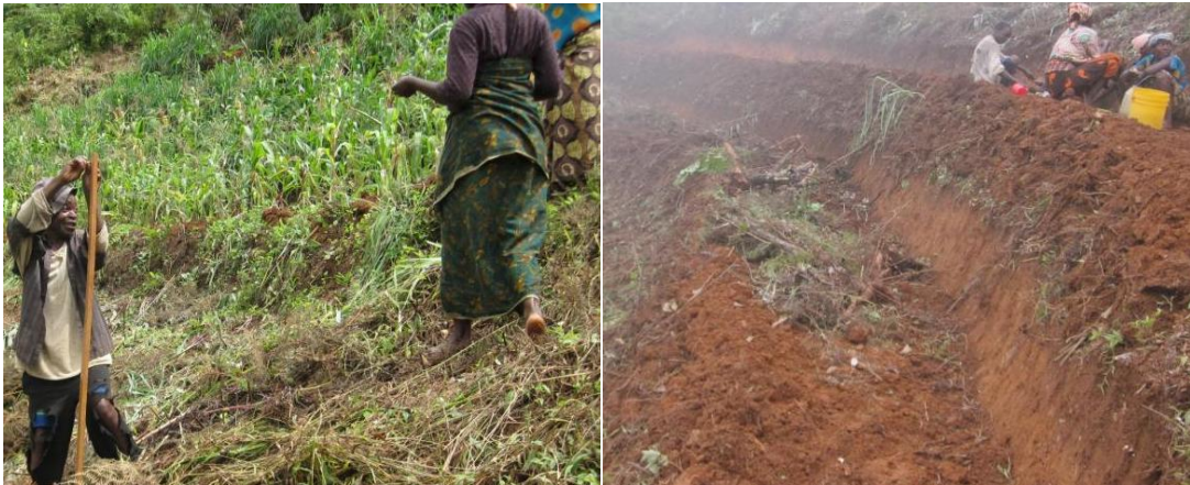
Figure 3.5. The construction of bench terraces in progress as found in Kibungo village. The left plate shows farmers taking measurements and the right plate shows the constructed bench terraces.
