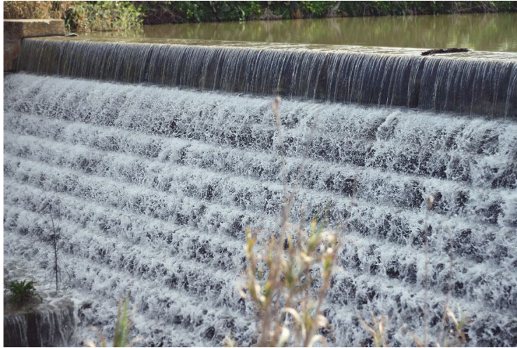
Figure 53 Overflow of water. When the lake is full water cascades from one reservoir to the next.
