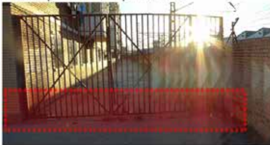
Stage 22- Security gate to stop access to the back street. The interface area shows the device, privatising what it was originally the street.
