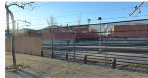
Stage 21- Edge between street and railway line. Brick wall, metal fence and bollards
